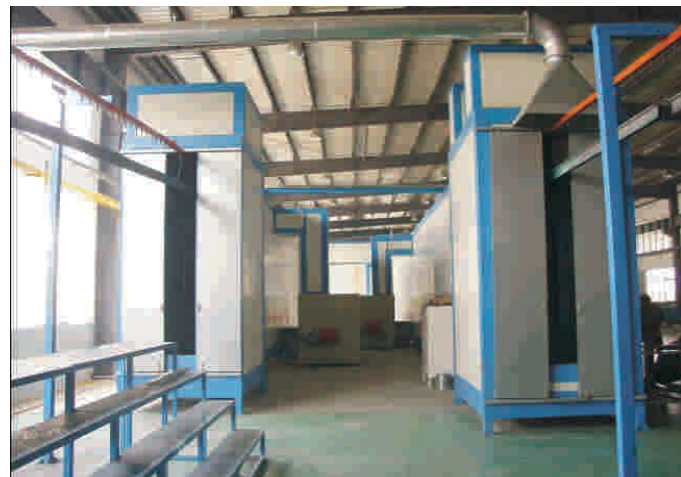
Dry off oven & curing oven
