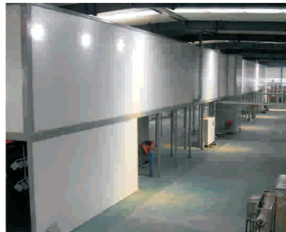
Tunnel type powder coating curing oven
